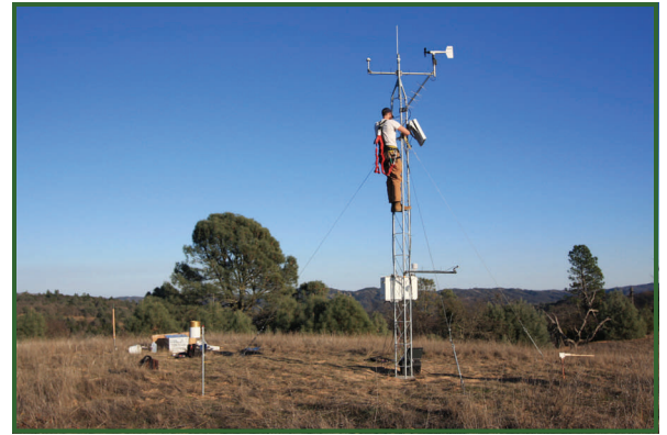
Installation almost complete Photo by Dr. Craig Clements
