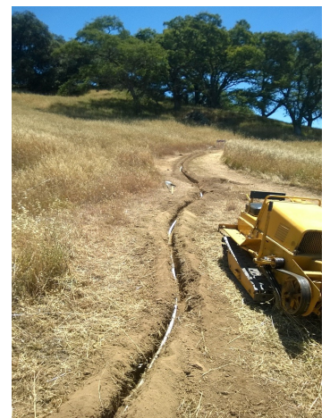
Coit Spring pipeline
